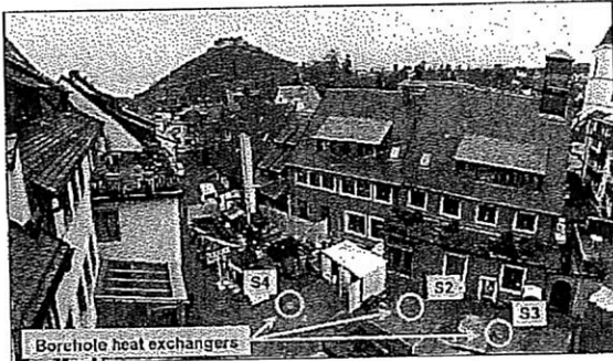
Fig. 12: Borehole heat exchanger field at Rathausgasse with drill rig for the first exploration boring for determining the cause of damage (March 2009). Photo taken from the tower of the town hall by U. Burbaum.
